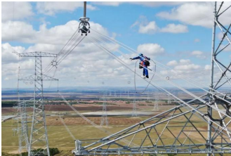
(c) Zhangbei-Xiongan 1000kV UHV Transmission Line.
